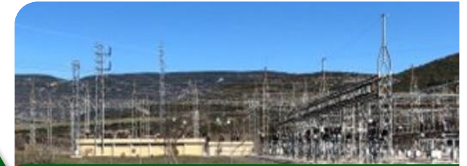
National Electricity Grid Substation in Sangüesa
