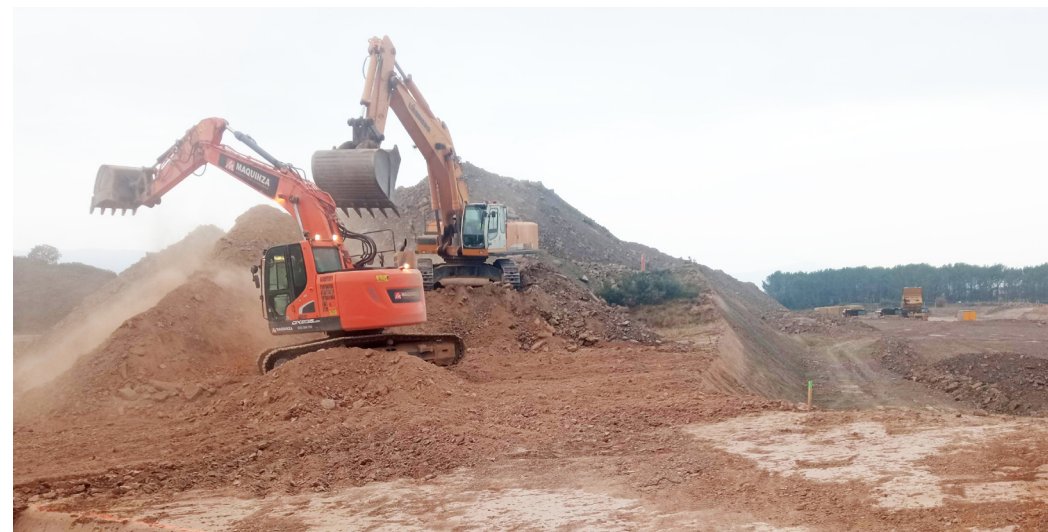
Preliminary construction activities at Muga involved mostly earthmoving works for preparation of the mine gate and declines
